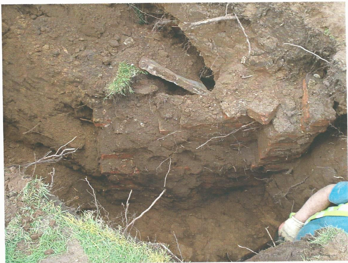
Pl. 80 Brick vault 606 after excavation of the trench around the west side, looking north
