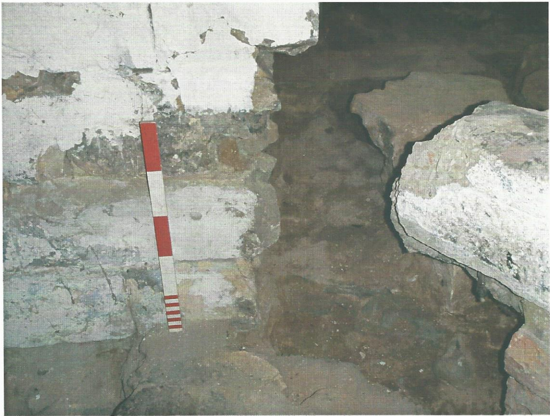
Pl. 67 Detail of north-west corner of opening showing damage caused by insertion of heating pipes, looking east. Scale 0.50m
