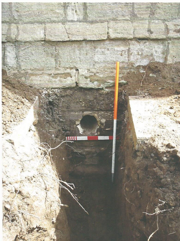
Pl. 84 Hole for service pipes in tower west wall. Scales 1m and 0.50m
