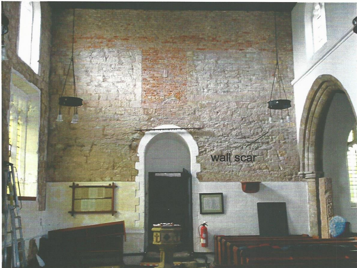
Pl. 16 Nave west wall showing wall scar for original position of the nave north wall
